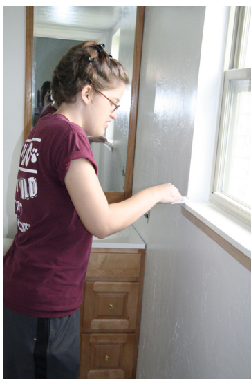
Michelle Fink works on some of the final touches in Friends Hall.
