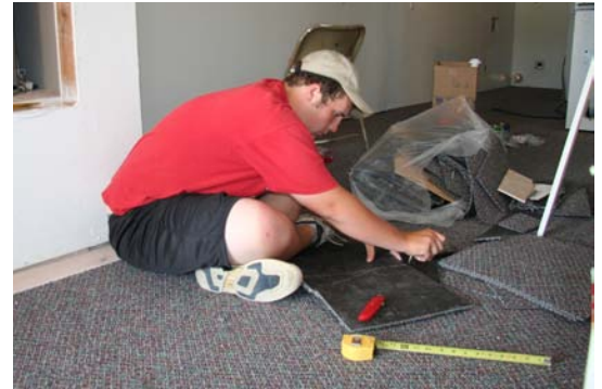
Ray Paxton lays new carpet in one of the dorm rooms in Friends Hall.
